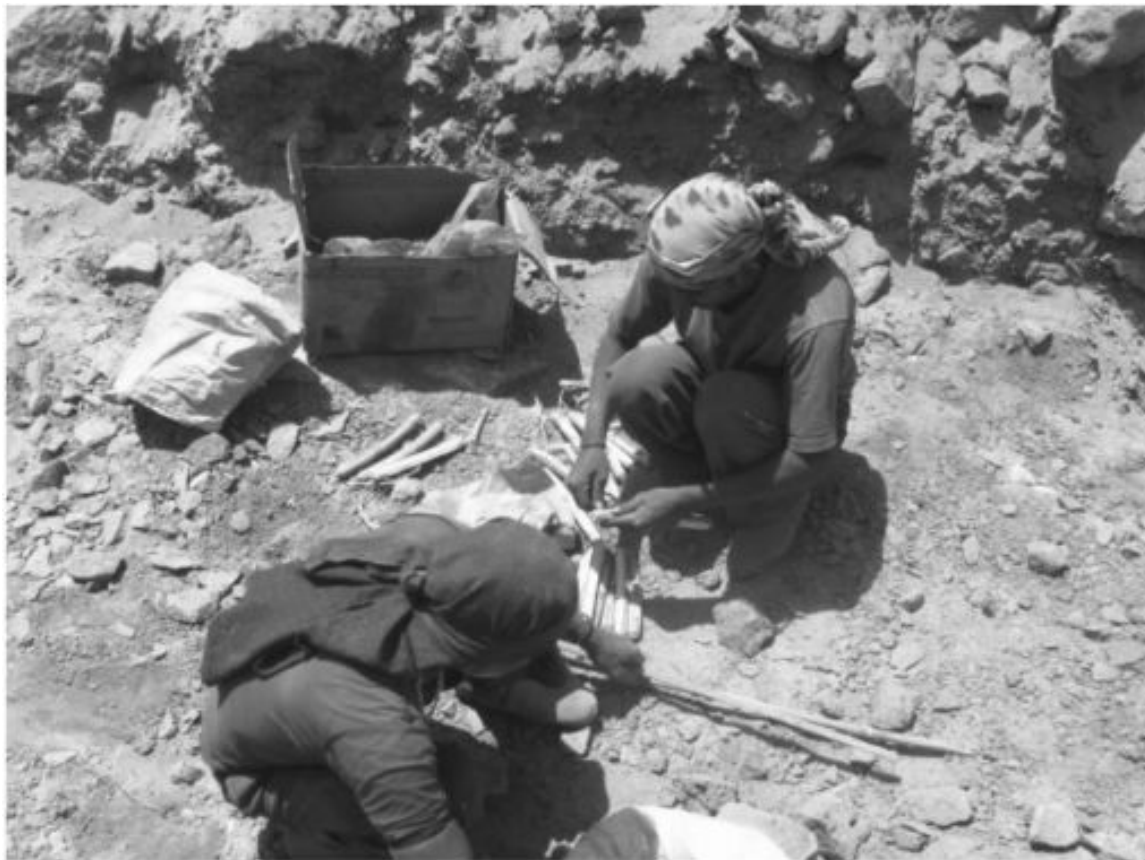
Figure 7.4 Labourers engaged in blasting activity for a 113 MW wind power project coming up in Maharashtra.
