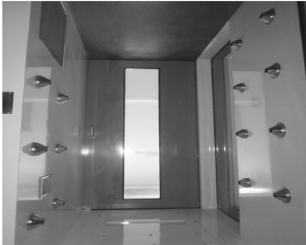
Figure 1.5 Air shower connecting Class 10,000 and Class 100 cleanrooms.
